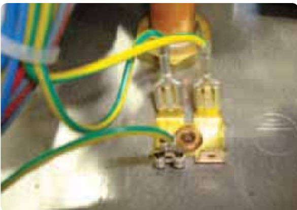
Figure 136 Ignition electrode grounding
