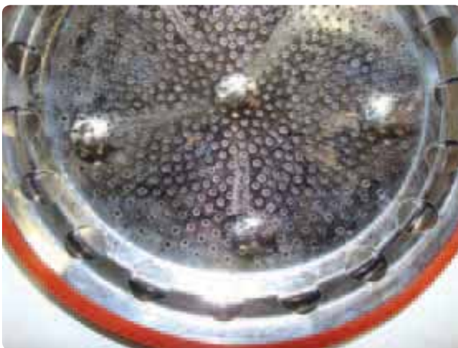
Figure 140 Inspecting interior and cleaning the burner
