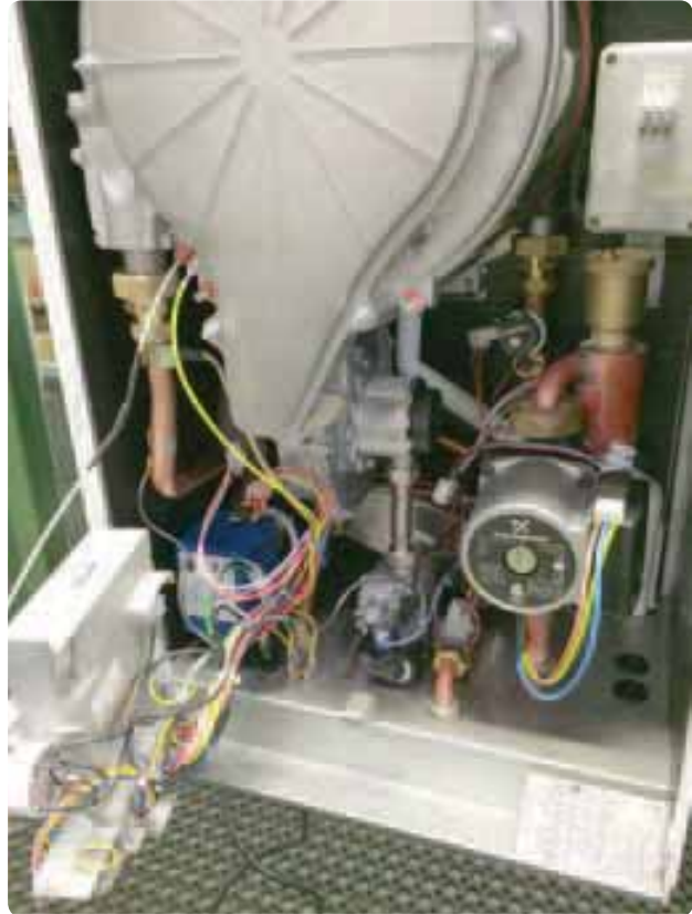
Figure 137 Boiler front panel removed
