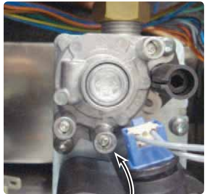
Inlet test port
