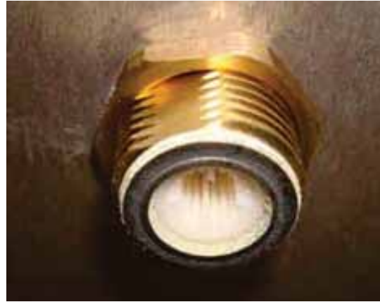
Figure 44 DHW inlet has a filter screen
