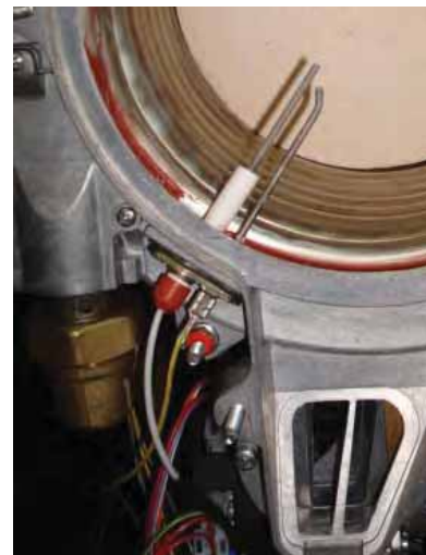
Figure 128 Inspecting ignition electrode
