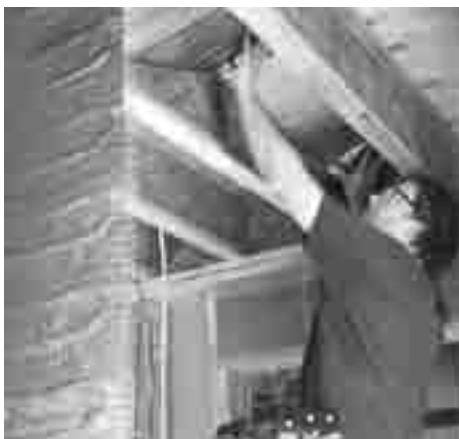
Test fit the mat between the joists before stapling the mat to the joists.
