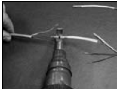
Step 2.13. Use a heat gun to carefully heat the solder ring (a red flux helps indicate this ring). Heat until the solder completely melts into the wires. If the solder is not completely melted, this connection will fail. Move the heat gun back and forth to continue heating the tube, shrinking it and melting the gray adhesive bands at the ends of the tube. Do not over heat the tube or the insulation on the wires, causing damage. Allow this solder tube to cool for about 1 minute.
