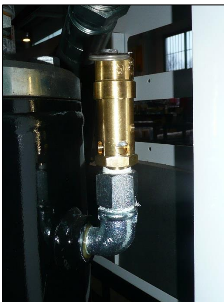
Figure 12.1-1 Control of the safety valve
