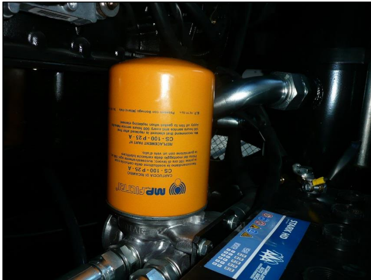
Figure 13.4-4 Compressor oil filter
