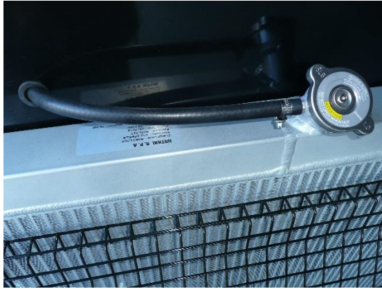
Figure 10.1-3 Checking the radiator cooling liquid
