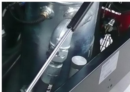
Figure 10.1-1 Checking the oil level in the compressor
