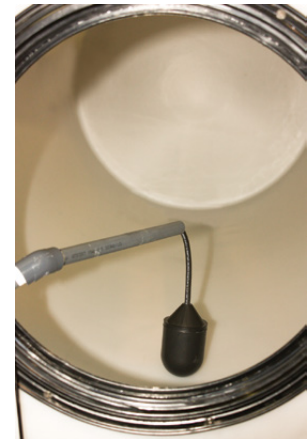
Pre Installed Float Switch
