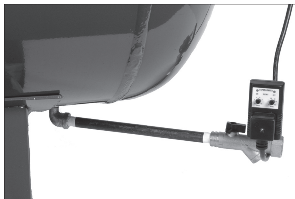
Figure 17 - Automatic Tank Drain
