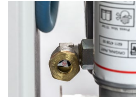
Oil level check
