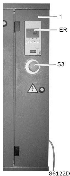
Control panel, Pack
